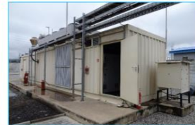
2 No. Emergency/ Black Start Diesel Generators 2.5Mva Each
