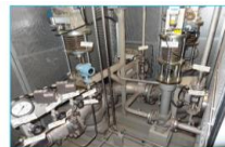
Control and Main stop valves Gas Skid
