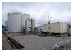
Raw Water Storage Tank for fire fighting and Demin Water Production
