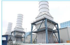
GT Exhaust Stacks Overview
