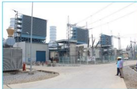
GT Overview with Filter Houses
