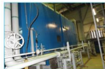
Water Cooled Generator TLR
