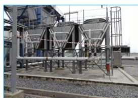
Bearing Oil Cooling Fans
